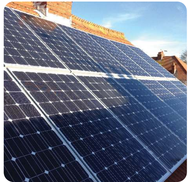
Figure 1. Solar panels in partial shade. Source: lowcarbonlivingblog.wordpress.com
